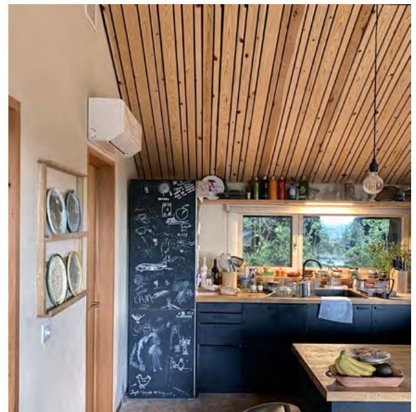
2.5 kW Mitsubishi minisplit installed at Old Holloway – sufficient to heat the whole building. Image: George Mikurcik
