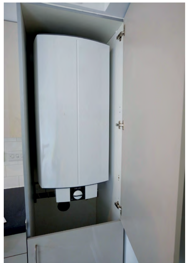
Water tank located in a cupboard. Photo: Alan Clarke
