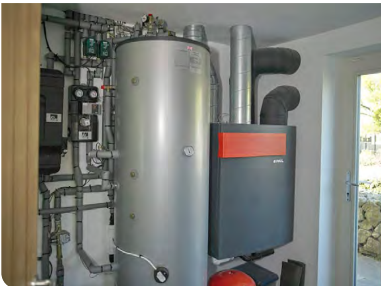
Plant room at Old Forge Cottage Passivhaus. Image: Green Building Store
