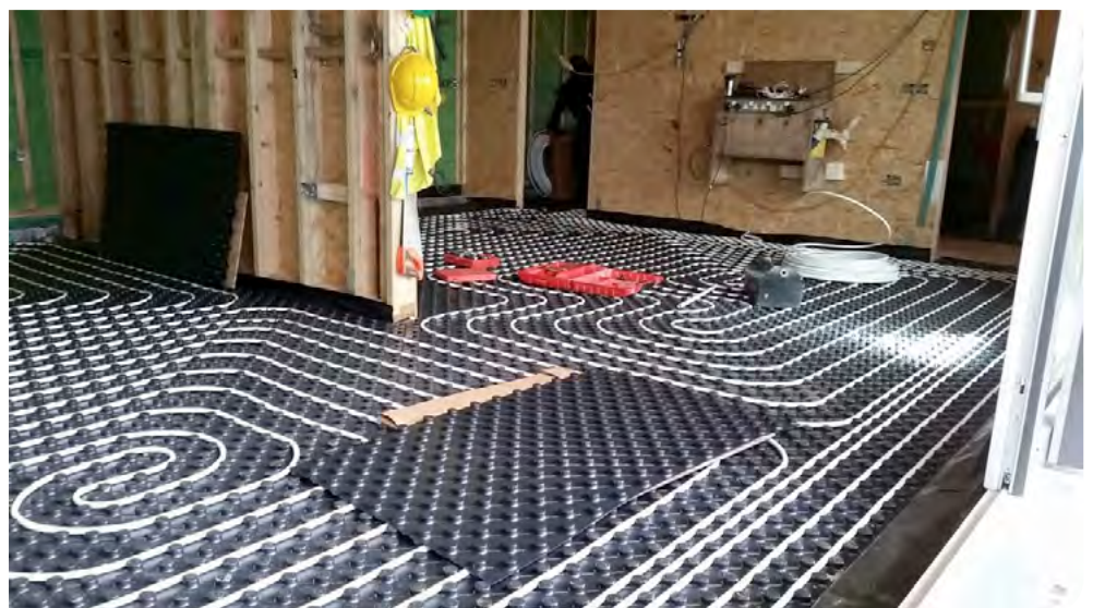
Underfloor heating at Bristol Passivhaus Plus. Image: Greenheart Construction
