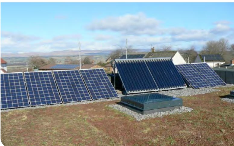
PV or solar thermal - or both? Renewables installation on a green roof at Ostro Passivhaus. Image: Paper Igloo
