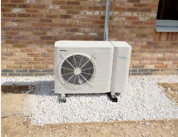
Air source heat pump. Image: Alan Clarke
