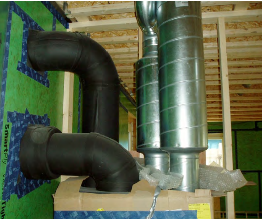
Above: MVHR unit during installation at Fishleys Passivhaus. Image: Liz Taylor and Mike Hill
