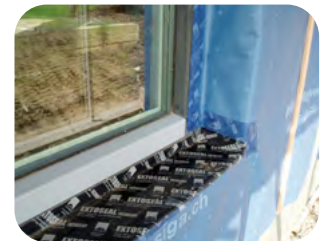
Air barrier installed in a manner that allows easy inspection and remediation during construction.
