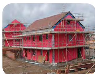
Wind barrier installed in a manner that allows easy inspection and remediation during construction.
