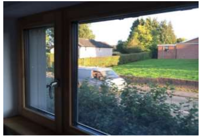
Figure 3. Bedroom window left closed due to busy road. Image Nick Grant.
